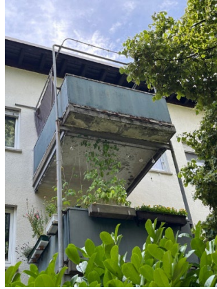
Picture 2: Poorly maintained housing stock managed by Vonovia in Frankfurt am Main.
