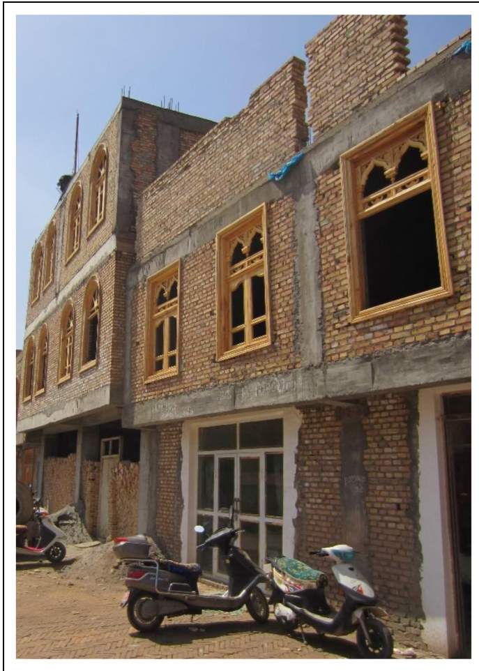
Figure 4. New “old” buildings being constructed from scratch, Kashgar 2014. What can be seen at this stage is that though the window frames are carved in the traditional style, the buildings have concrete internal structures, and modern chrome and glass front doors. Officially to make them more earthquake-proof, this reconstruction is not a “conservation” of the original buildings, but a creation of a simulacrum of historic styles around/above a “modern” commercial building. © David O'Brien and Melissa Shani Brown.
