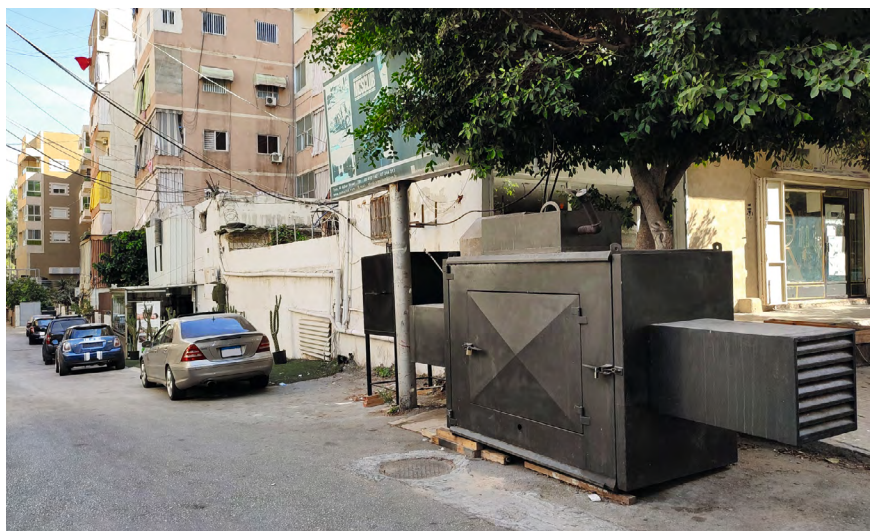
A private diesel generator at ground-level for alternative power supply at a street corner of Tyre, southern Lebanon. It runs and emits exhaust fumes for about 18 hours a day. Photo: Karim Eid-Sabbagh
