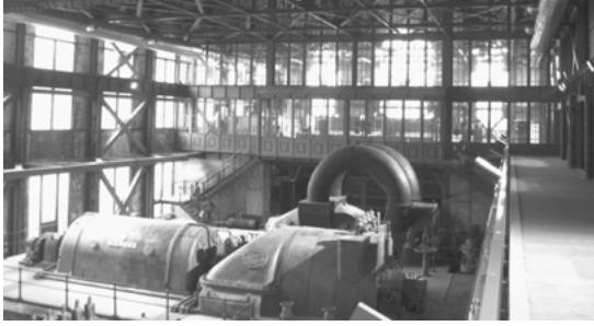
Figure 2: The interior of Museum of Energy former main power plant, photo by Senem Zeybeykoğlu.
