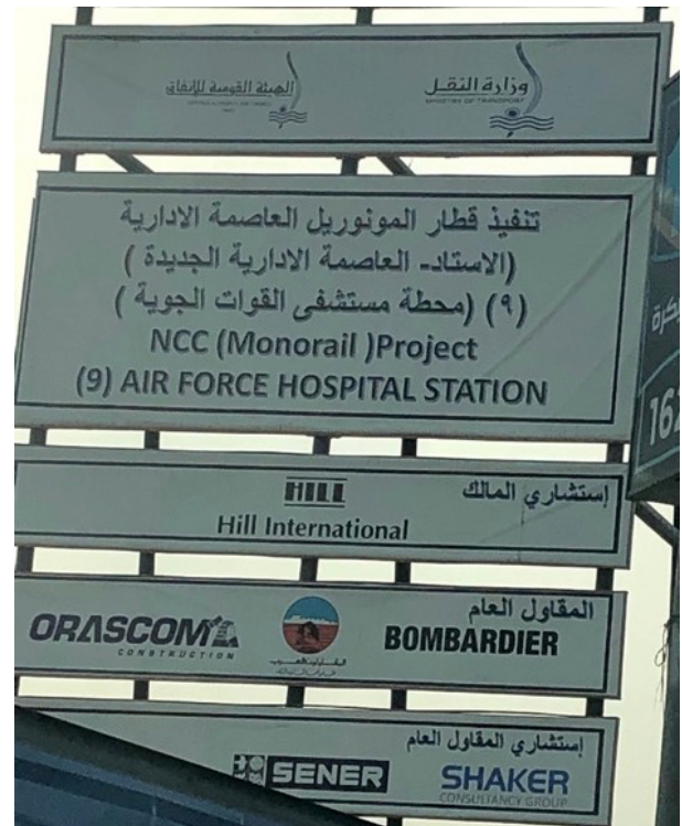
Figure 10. Monorail construction in New Cairo district. Note: Date: January 2021. Source: Safa Ashoub.
