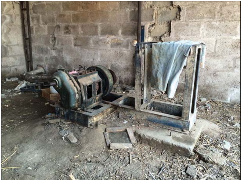
Figure 1. Broken Down Equipment
