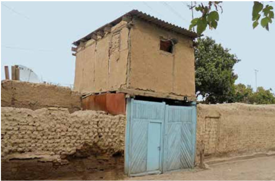
Photograph 1: Housing extension with loam: a bolo-hona ("on-top house") in Khujand's old town, Razzoq quarter, 2009 (Wladimir Sgibnev)
